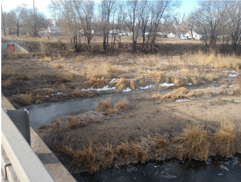
Figure 5 – Significant Sediment Deposition Exists west, east and under Highway 85 Bridge
